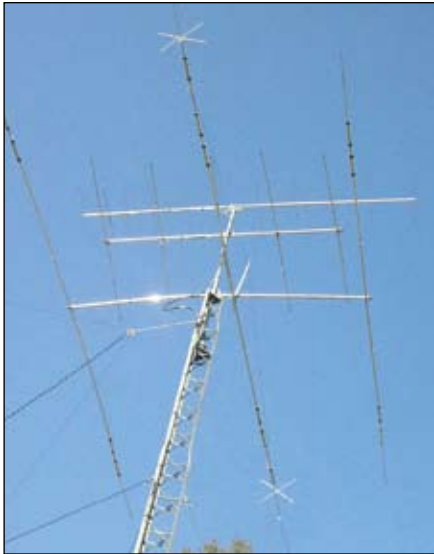
The antennas at WK4P. The tribander and wire did all the work this time.
